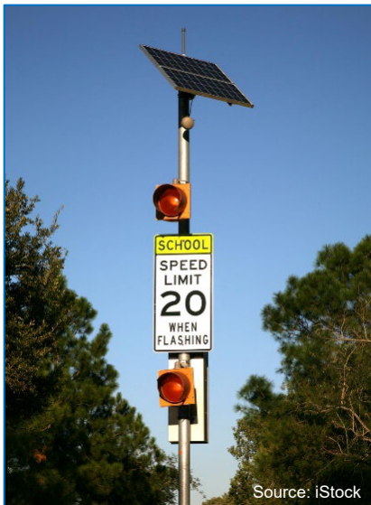
Figure 3: A typical pedestrian flashing beacons. Source: iStock
