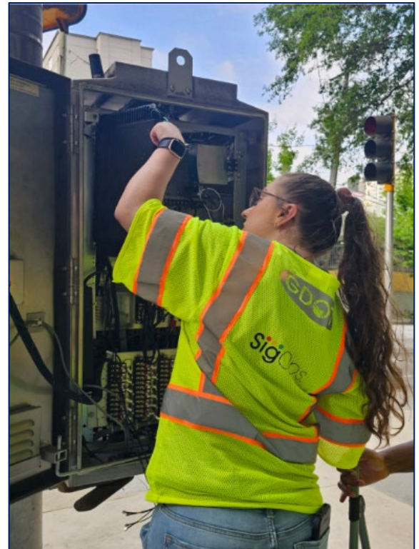
Figure 3: Georgia DOT deploying Palo Alto Networks PA-450 series firewalls to secure edge network communications, enhancing cybersecurity across the state's transportation infrastructure (Source: NOCoE)
