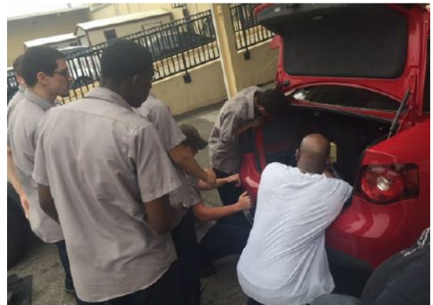
Figure 3. Students from Hillsborough Community College's Master Mechanic Program work to install the CV equipment in Pilot participants' vehicles. Source: THEA
