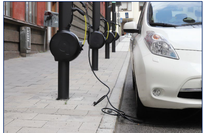
Figure 2: Curbside EV charging stations (Source: iStock).
