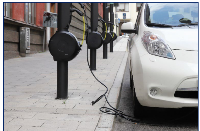
Figure 2: Curbside EV charging stations (Source: iStock).
